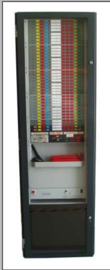
Master Control Panels (MECP)
